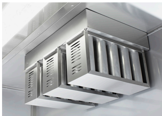
The cyclone filter's measurement socket is located at the top left of the filter housing
